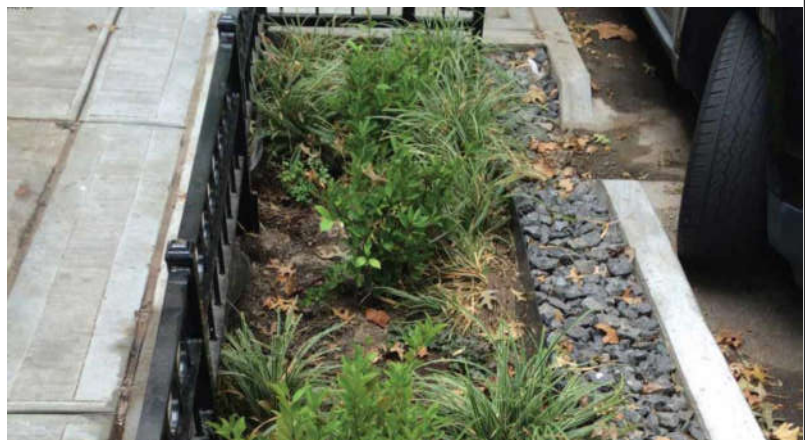
Street-side bioretention planter located in New York. Source: National Association of City Transportation Officials
